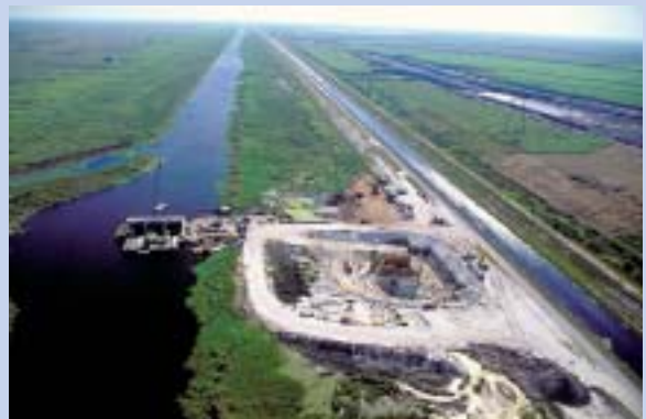
The inflow and water distribution works for STA 1 (stormwater treatment area), which is a large constructed wetland that is treating runoff from sugar cane fields before entering the Everglades. Photo from the South Florida Water Management District archives.
